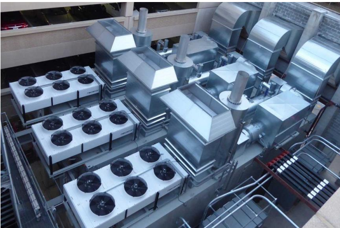
Three 2G Energy - 2 MW Feb 11 Packaged CHP Systems SOURCE: UNISON ENERGY
