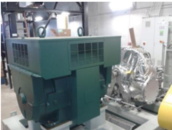
Backpressure Steam Turbine/Generator Photo courtesy of Gundersen Health System
