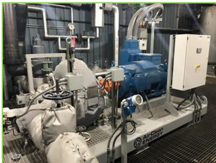
Hancock Lumber’s 300 kW backpressure steam turbine
