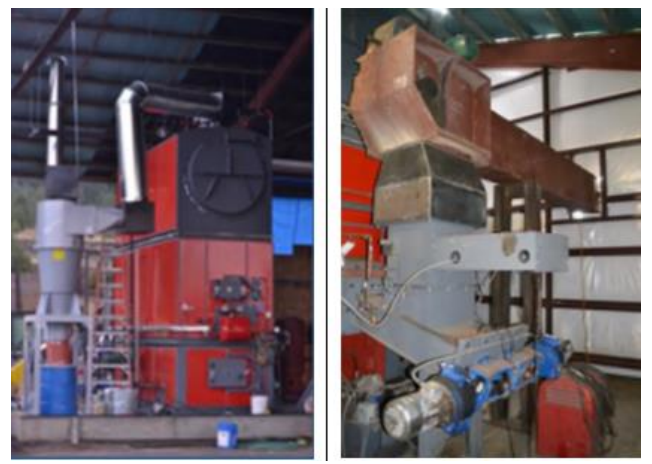
The 4.7 MMBtuh Uniconfort biomass gasifier (left) and the in-feed from the wood chip bin (right)
