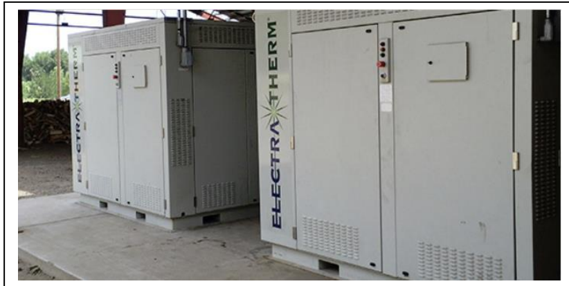
Two 50 kW ElectraTherm+ 4400 Organic Rankine Cycle “Green Machine” power generators.
