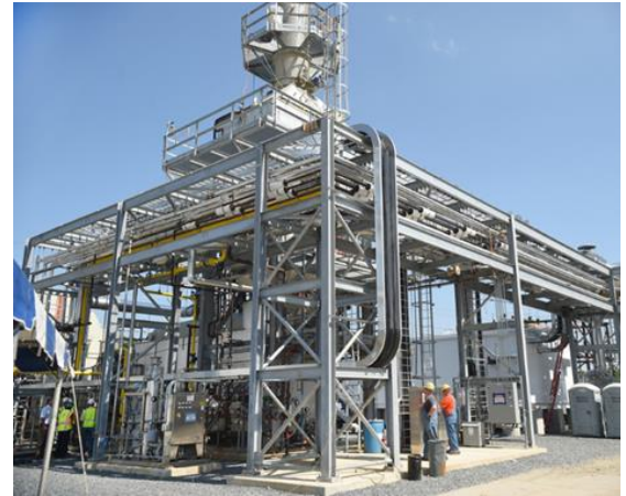
7.9 MW combustion turbine generator at Aberdeen Proving Ground
