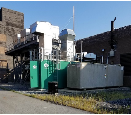
220 kW Packaged CHP System
