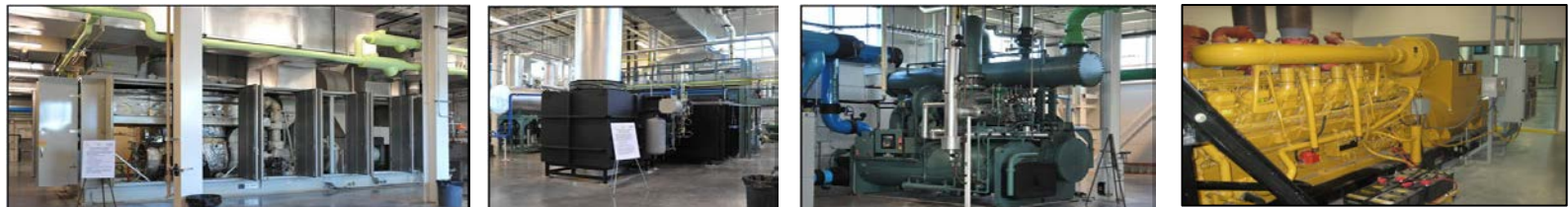
CHP System Equipment: Gas Turbine, Heat Recovery System, Chiller, Backup Generator
