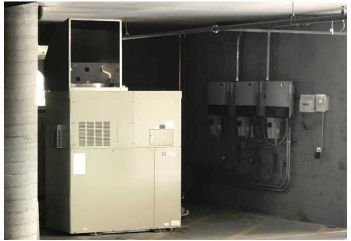
The CHP installation at the Towers II student housing complex consists of 10 kW and 5 kW packaged natural gas-fired Yanmar reciprocating engines.
