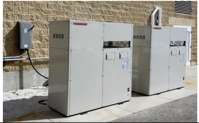
Two 35 kW Yanmar reciprocating engines in outdoor enclosures.
