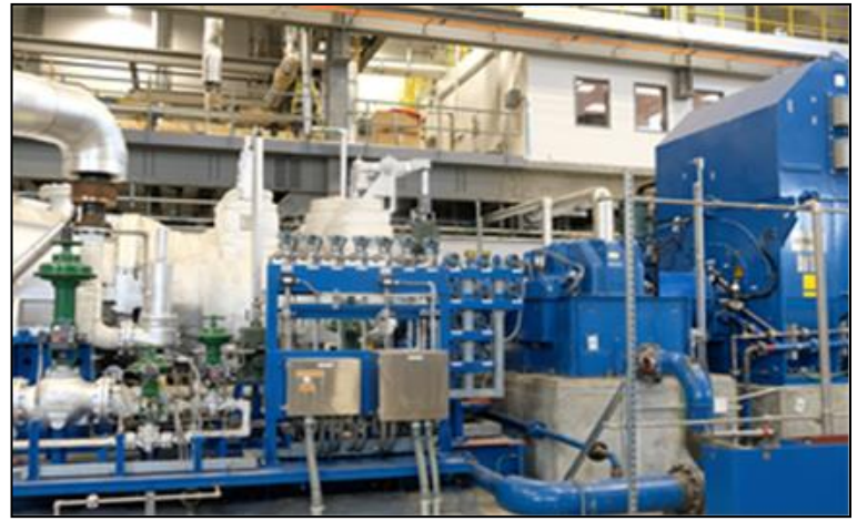
The 17 MW Extraction/Condensing Steam Turbine
