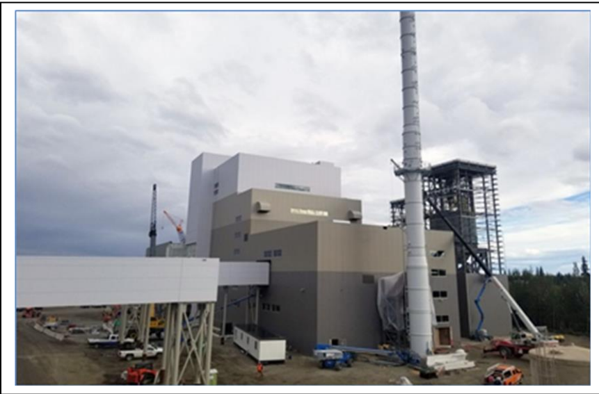
The New University of Alaska Fairbanks Coal-fueled CHP power plant
