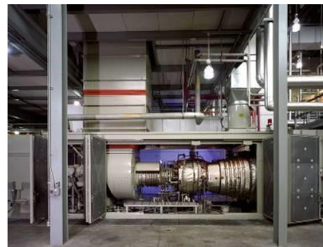
Gas Turbine Generator Photo Courtesy of University of Missouri
